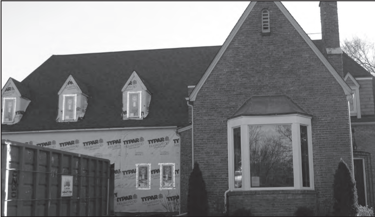
Peter Scholl's 1,800-square-foot addition to a landmark house in Crystal Lake was a garage with a second-floor master suite connected to the original structure.
